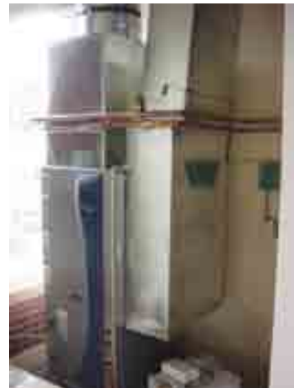
An air handler for a GSHP can be added to an existing central heating system.
