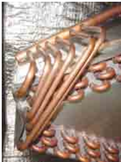
Inside the air handler (aka "air coil"), which is analogous to a car's cooling radiator coil.
